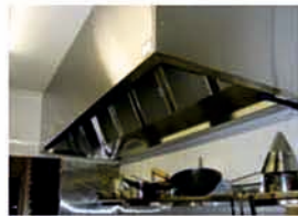
CENTRE EXHAUST HOOD
